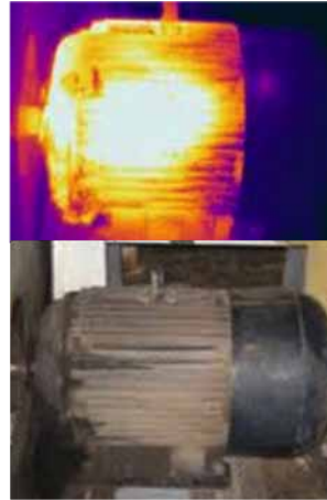
Figure 20: DOL motor failure due to overheating caused by negative sequence harmonics
