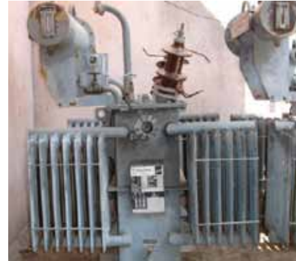
Figure 14: Overheating of transformers can result due to the presence of harmonics
